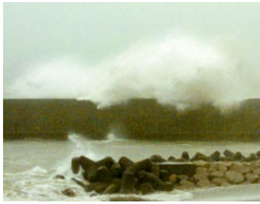
Tetrapods in action during a July typhoon that hit Kyushu. Photo by Aoyama Ken
