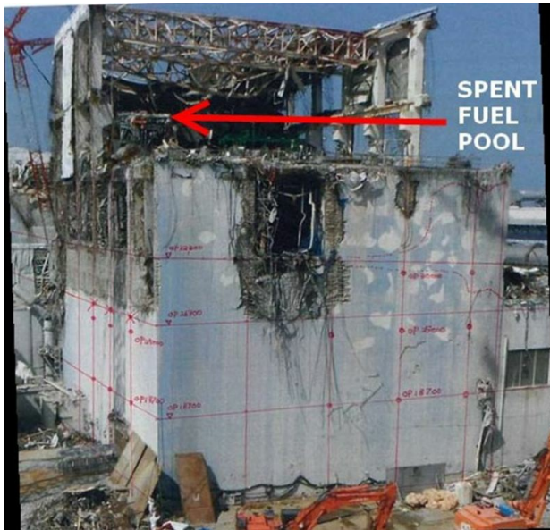
Spent fuel pool at reactor # 4 after the blast
