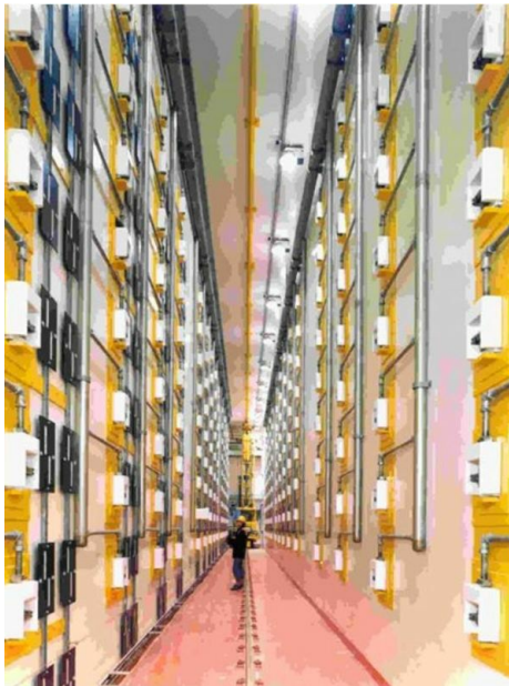
Plutonium storage area, Sellafield, England
