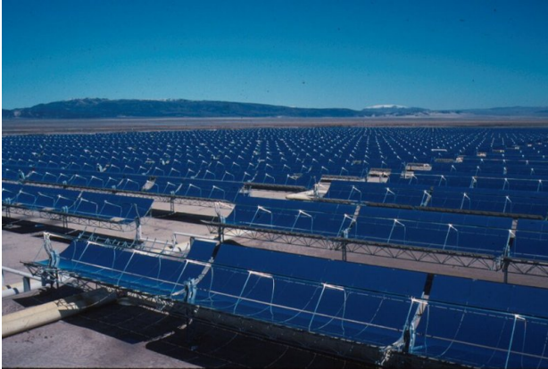
Dunhuang Solar Plant
