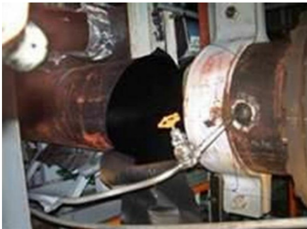
Pipes at aging Mihama reactor ruptured, releasing steam that killed four and injured seven in 2004
